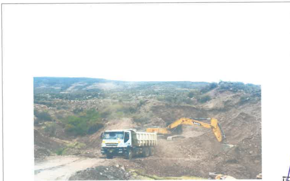
Fig. 02 Acarreo material granular (17L 784791E 9072326N) Alt. 3569.00m
