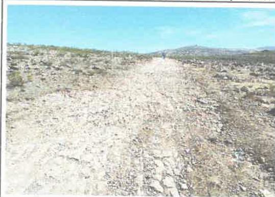
foto 01: KM 00 + 200, Deformacion - Erosion - Baches
