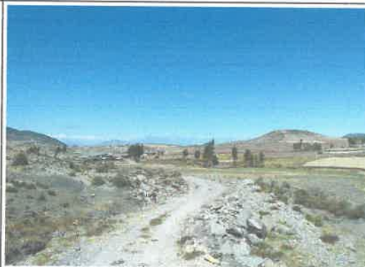
Foto 16: KM 9+450al 10+250, Erosion - Baches
