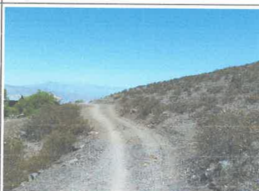
Foto 30: KM 12+750 al 13+800, Erosion - baches
