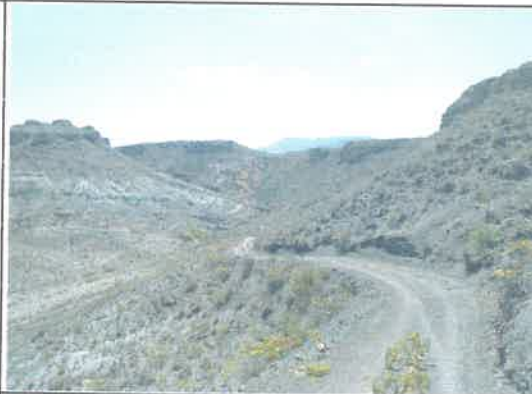
Foto 24: KM 11+700 al 12+250, erosion -Baches
